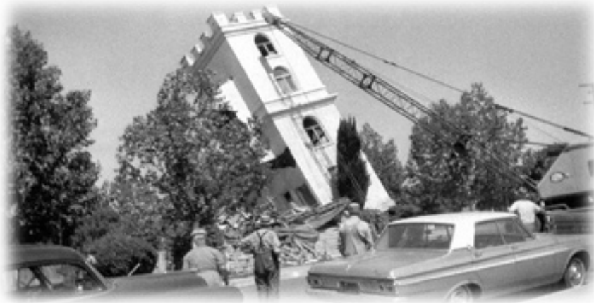
The south tower of the Reedley Mennonite Brethren Church falls during demolition of the building in July, 1965.
